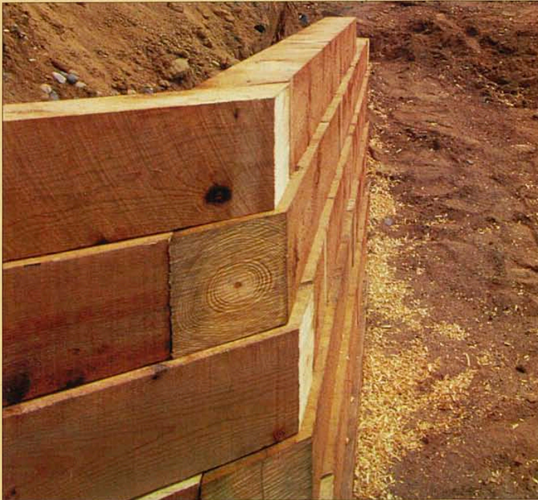
Tilting the wall toward the slope makes it strong. Johnson sets each course of timbers \frac{3}{4} in. back from the course below.
