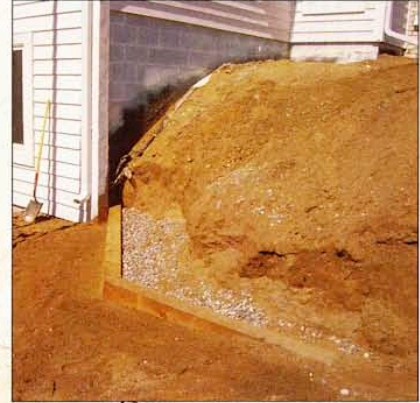
Timber walls need good drainage. Johnson installs 4-in.- to 6-in.-dia. perforated pipe along the footing and shovels 1 1/2-in. gravel against the timbers.
