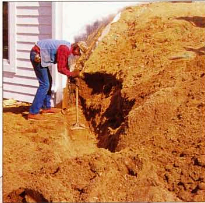
Timber retaining walls demand careful construction. If the bottom timbers shift or settle, so will the wall. Author Johnson digs a trench for them, and levels and compacts the soil, as shown here.
